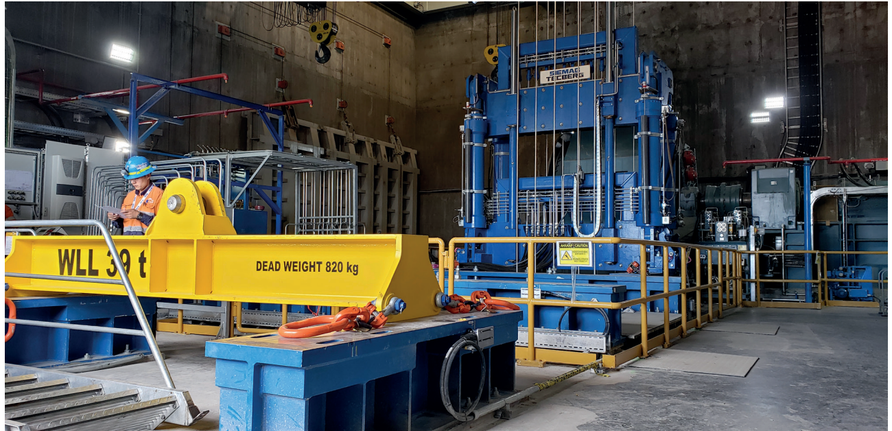
Installation of the 6-rope clamping and lifting device (CLD) in shaft 2 of Oyu Tolgoi.
