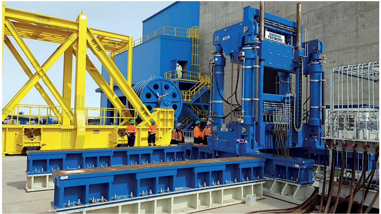
Preparations for rope laying: Assembly and functional tests of the equipment. On the right in the picture the 6-rope clamping and lifting device with hydraulic system.
