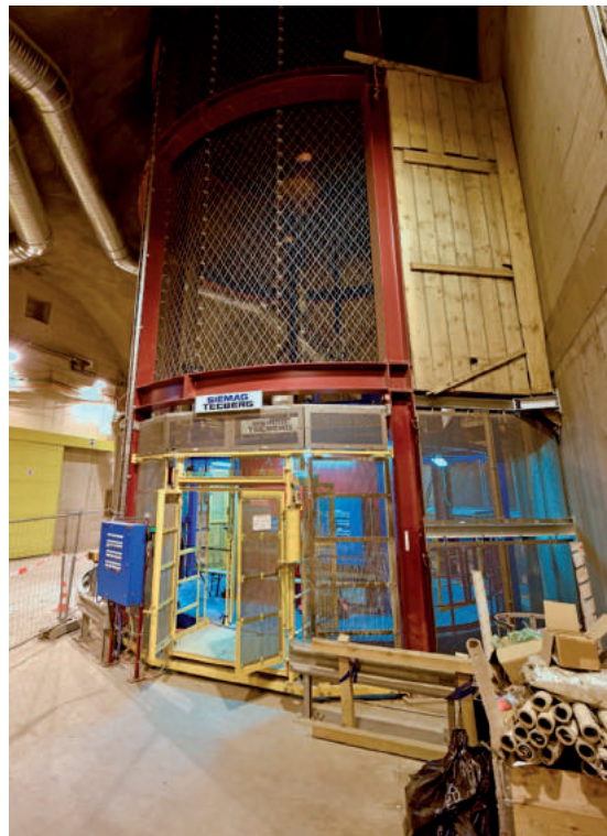
Fig. 13: Shaft station steelwork with shaft access gate, call bell system, removable access panels and high-tensile wire mesh screen
