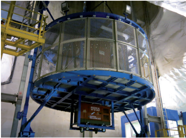
Fig. 4: Inspection platform as medium-sized manriding system with pluggable access panels in parked position
