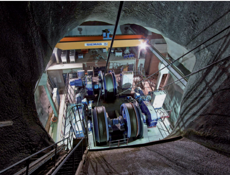
Fig. 7: View from the rope channel of the shaft hoisting systems for the GBT operating phase
