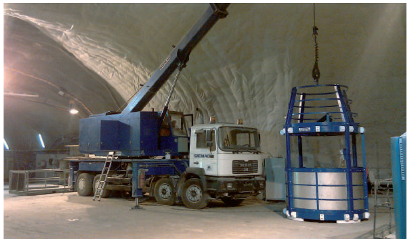
Fig. 6: Mobile shaft winch with inspection cage for Shaft II
