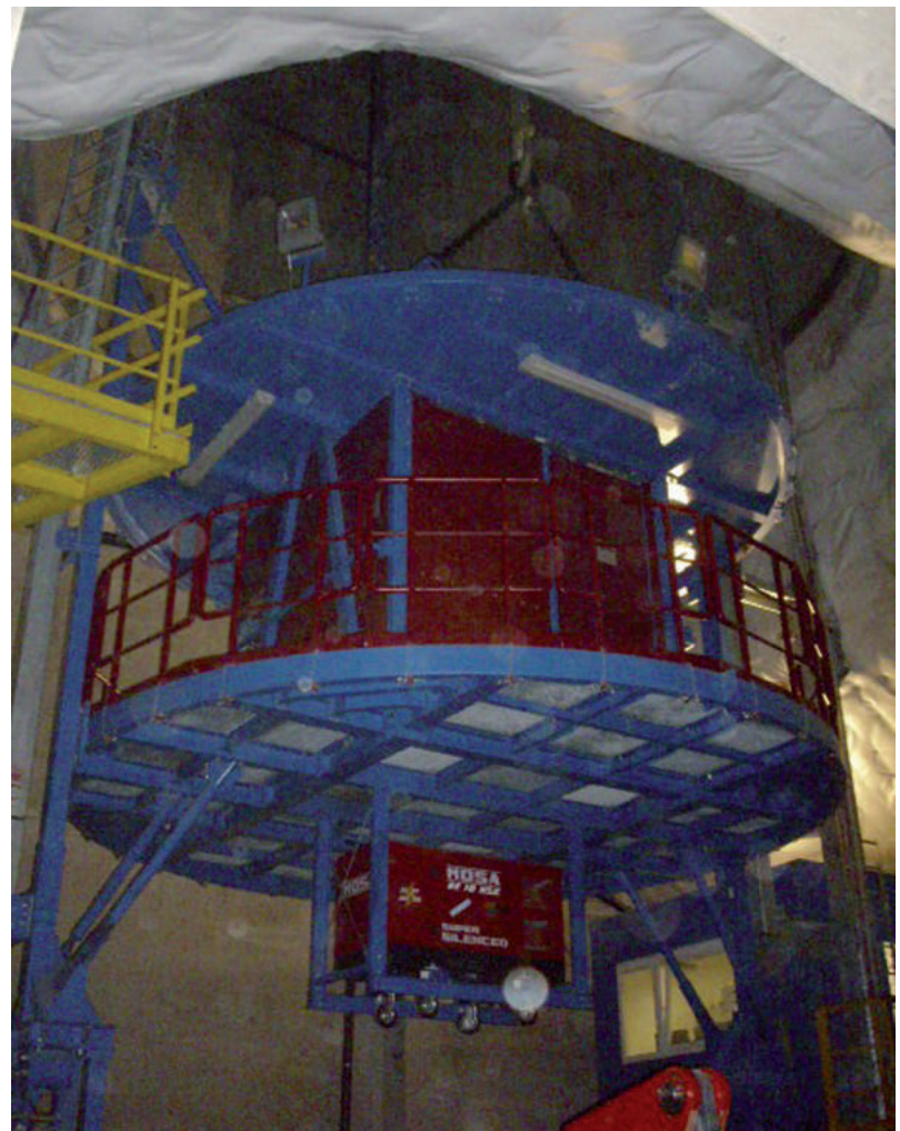
Fig. 3: Inspection platform (IPF) as maintenance platform with pluggable railings in parked position
